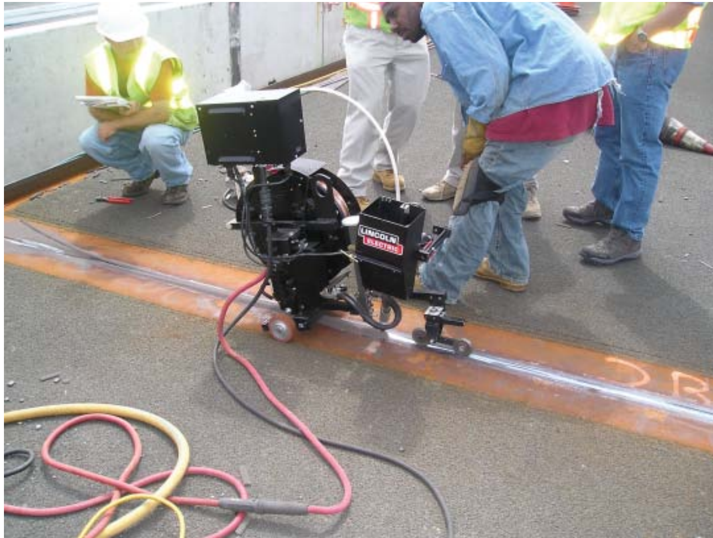
ABOVE Workers operate a submerged arc welding machine, joining the new deck panels.
