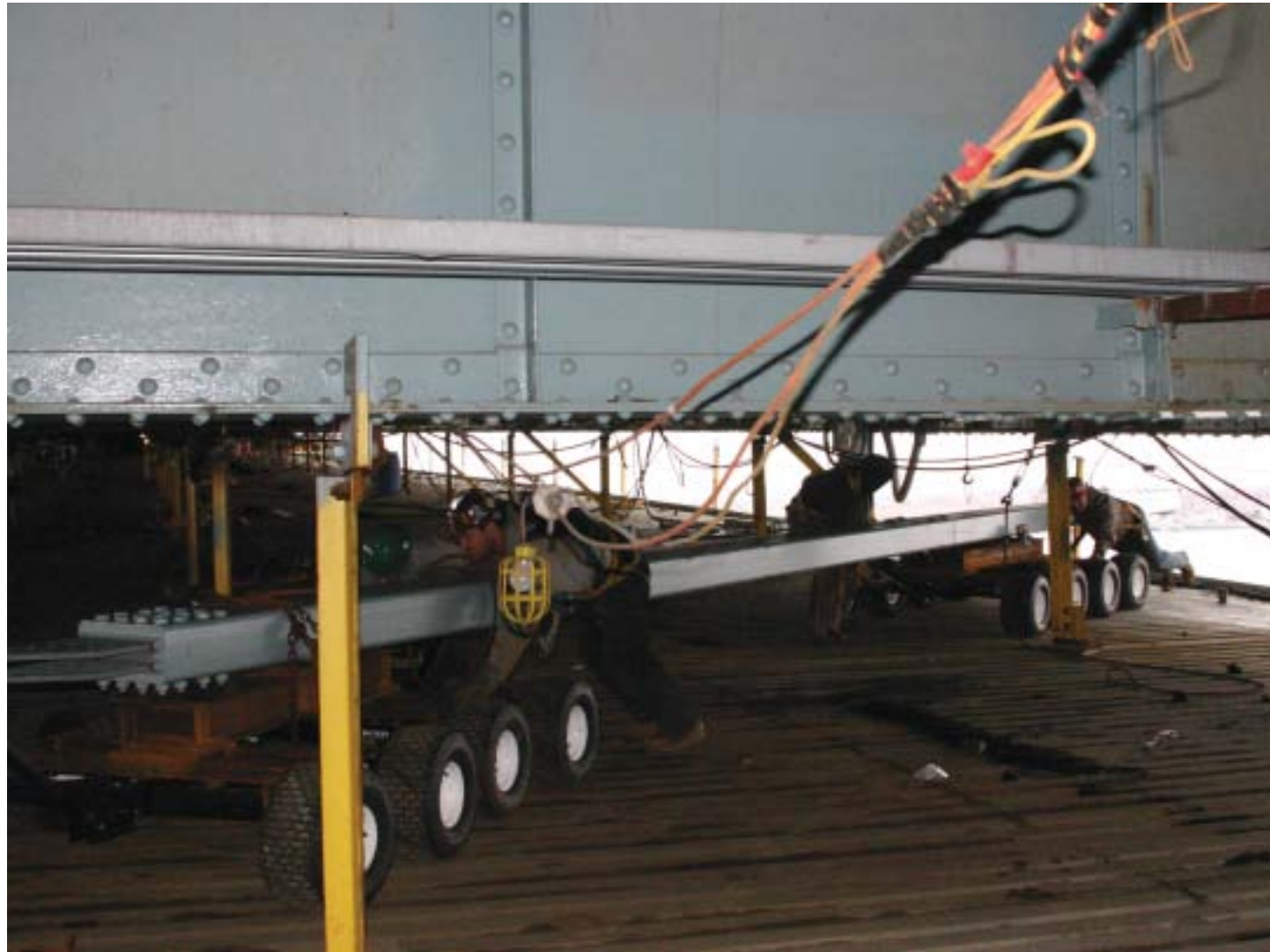
ABOVE Ironworkers maneuver the new lateral system into place on a temporary construction platform beneath the bridge.
