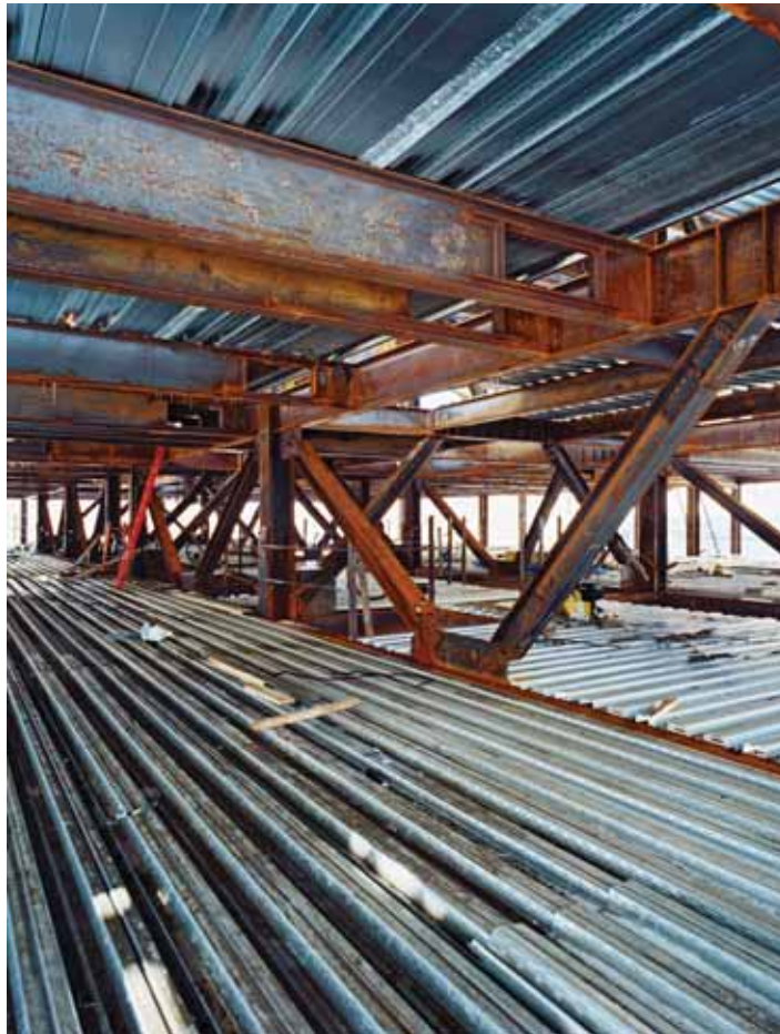
ABOVE AND OPPOSITE Running HVAC through penetrations in the structural steel girders allowed the designers to maximize ceiling heights.
