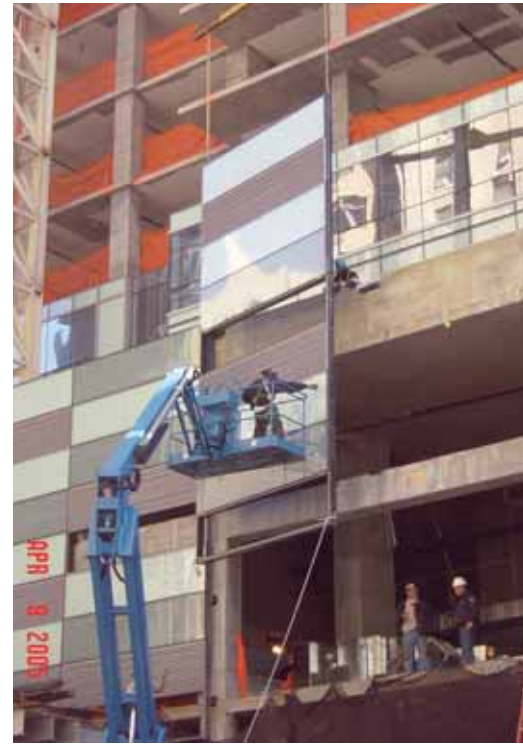
BELOW This system is erected clockwise or counterclockwise around each floor, rather than by elevation.
