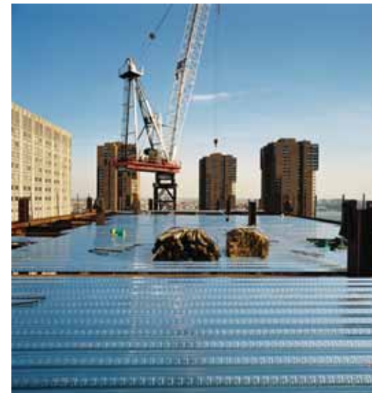
TOP Before pouring the floor, the steel deck was reinforced and outfitted with electrical conduit.
