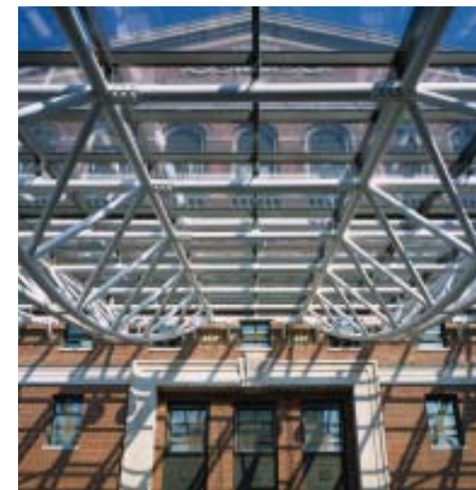
ABOVE The bow trusses, fabricated from 6-inch XXS pipe, support a skylight of Viracon laminated glass.
